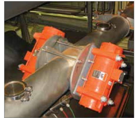
Consistent material flow is maintained by dual units in this pipe line.
