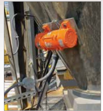
2PX surge bin application.
