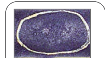
Hose with cover charred area from high heat or extreme aging due to heat or ozone
