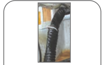
Crushed vent ducting, will impede proper and safe venting of fumes. Replace damaged duct
